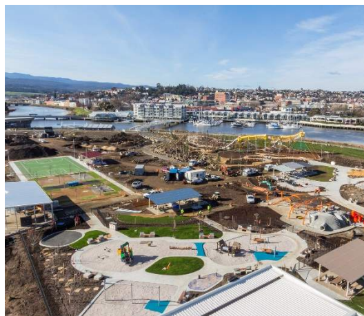
Project: Riverbend Civil Works Location: Lindsay Street, Launceston Client: City of Launceston Value: $2.5 Million
