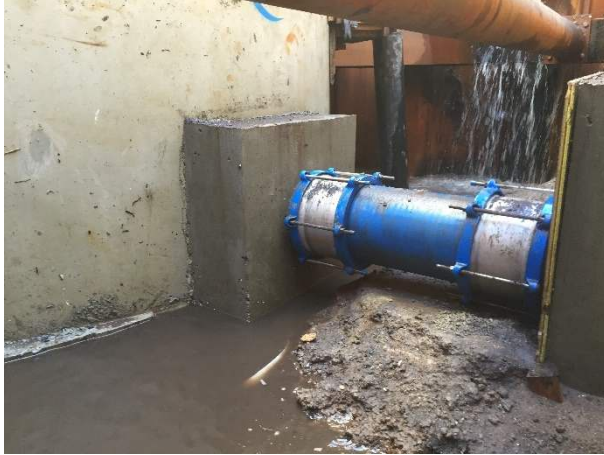
Project: Hobblers Bridge Sewer Main – 450 mm Location: Queechy Client: TasWater Value: $450k Client: TasWater
