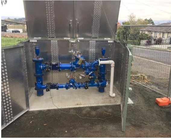
Project: PRV Install and Commissioning Location: Riverside & St Leonards Client: TasWater Value: $200k
