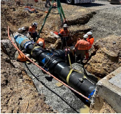
Project: 600 Dia Bulk Transfer Water Main Location: Mt Leslie WTP Client: TasWater CDO Value: $250k
