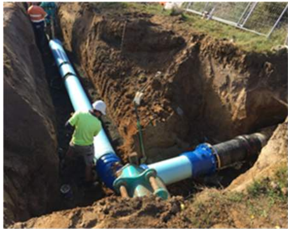
Project: 28 km, 300 dia. Water Main Location: Mount Direction to Lilydale Client: TasWater Value: $3.0 Million
