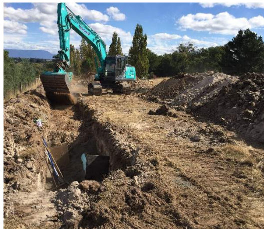
Project: 12 km, 300 dia. Water Main Location: Longford to Cressy Client: TasWater Value: $2.5 Million
